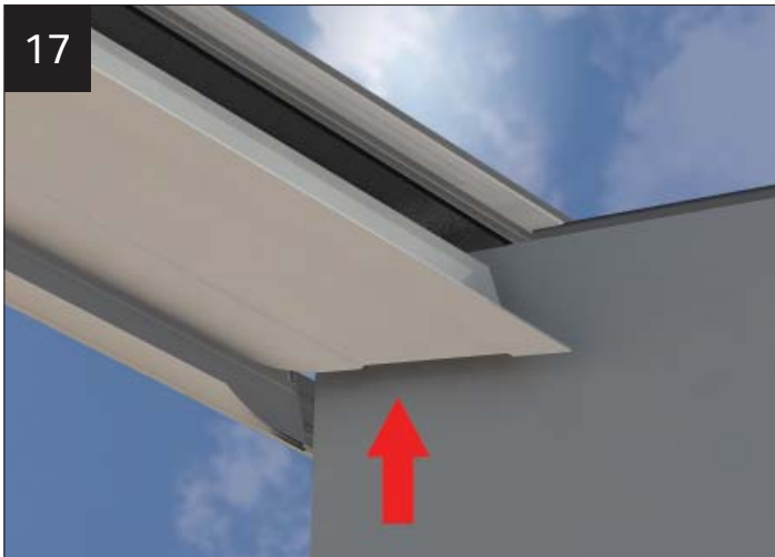
Classic Plus Valley cladding being fitted against pelmet. After plasterboard and skim.
