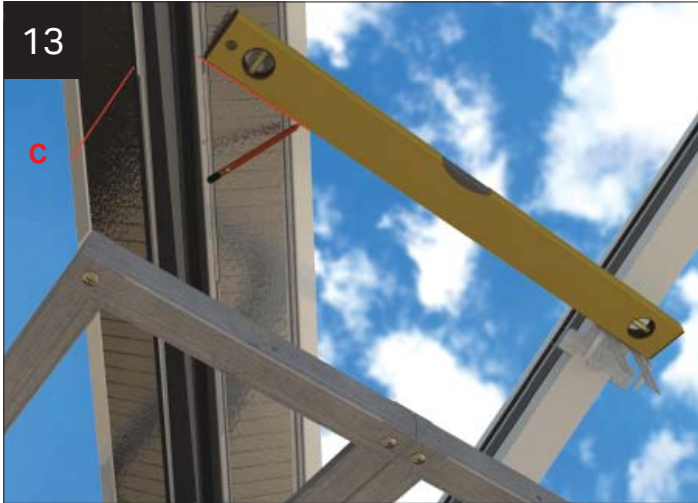
Using the bracket positions, level through and mark off the valley marked 'C'.
